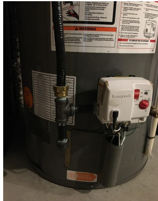
Water heater gas piping
