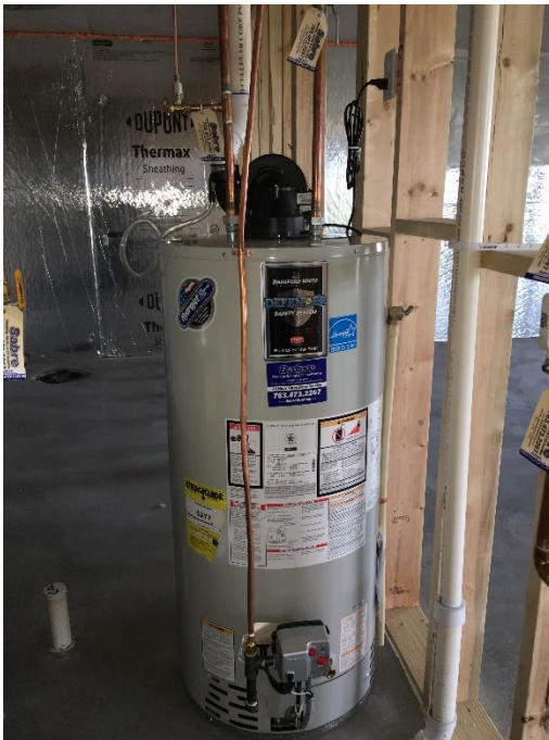
Water heater front view
