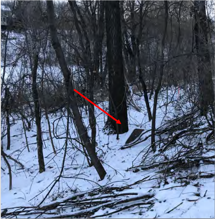
(Above) Pond outlet prior to improvements.
